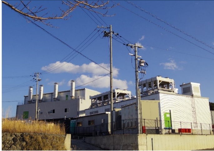
Shingu Forest Energy CHP 1.8MW
