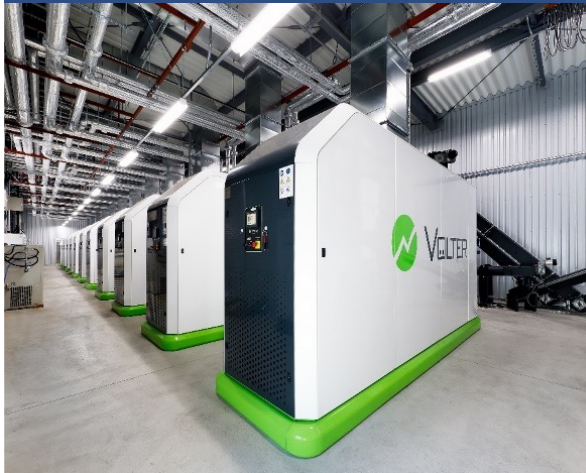
12 units of small CHP
