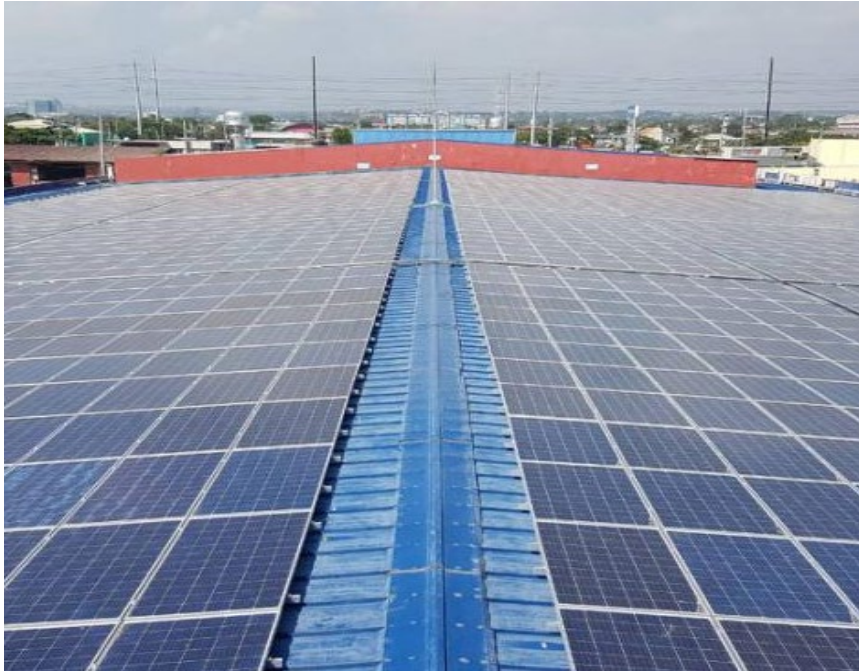
1100 kWp Solar Rooftop Project
