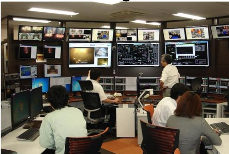
WtE (Waste to Energy) Plants remote monitoring room
